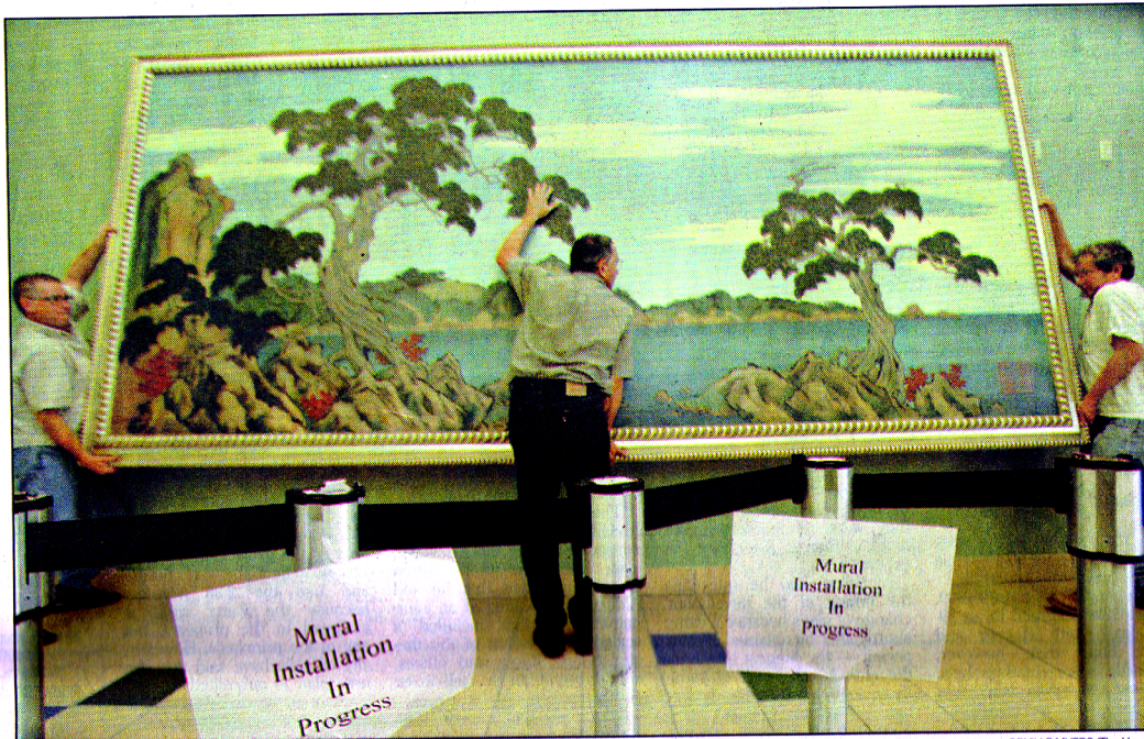
From left, Chris Botta; Jim Alkons of Northern California Art Conservators; and Gary Dinneen hoist the "Point Lobos" mural into place at CSUMB on Monday.
